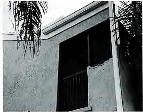
Photograph 12: Unit 208. Exterior wall opening
