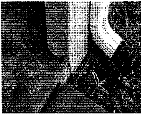
Photograph 9: Corner crack on exterior wall near downspout
