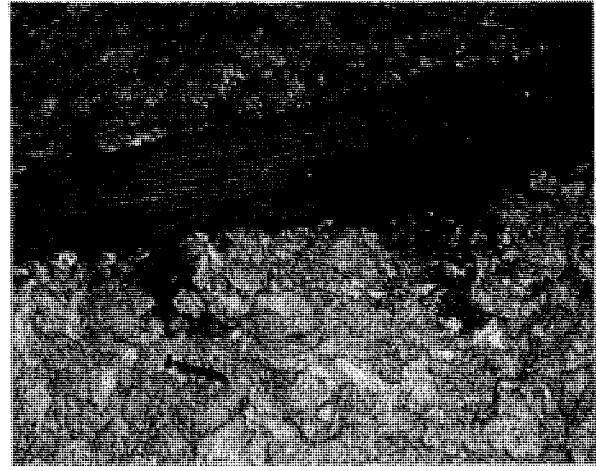
Photograph 14: Unit 208. Termites Infestation
