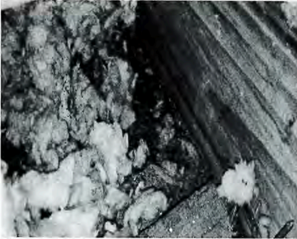
Photograph 13: Unit 208. Termites infestation
