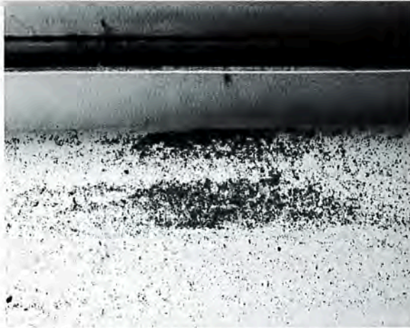
Photograph 13: Unit 208. Termites infestation
