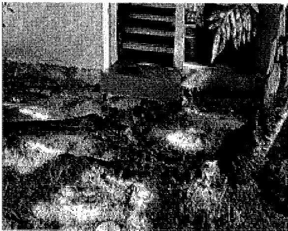
Photograph 9: Tree roots growing under foundation and soil washout
