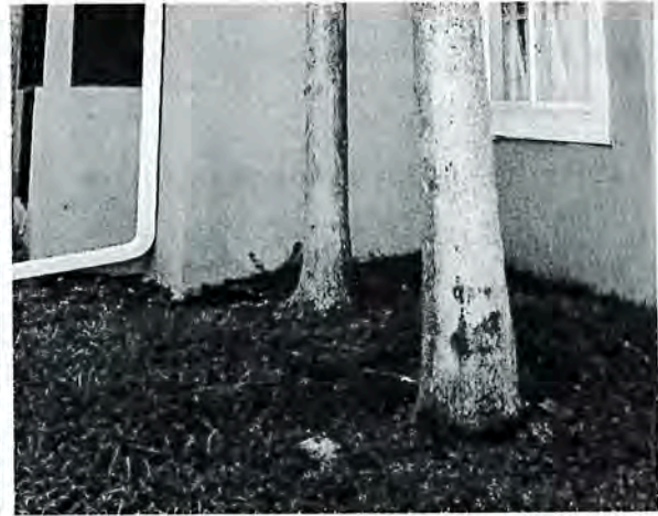
Photograph 14: Tree roots growing against the foundation
