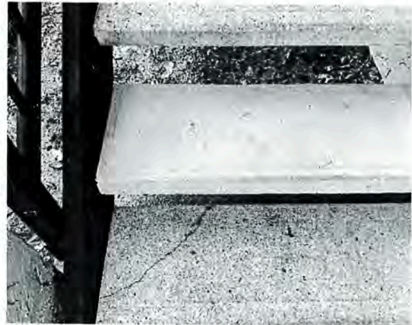
Photograph 18: Common staircase cracked concrete step
