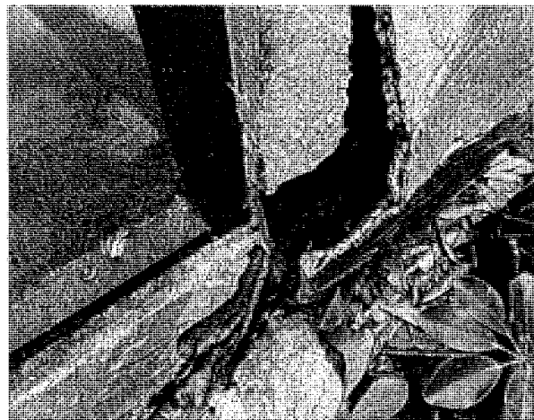
Photograph 4: Unit 105. Opening in the exterior wall
