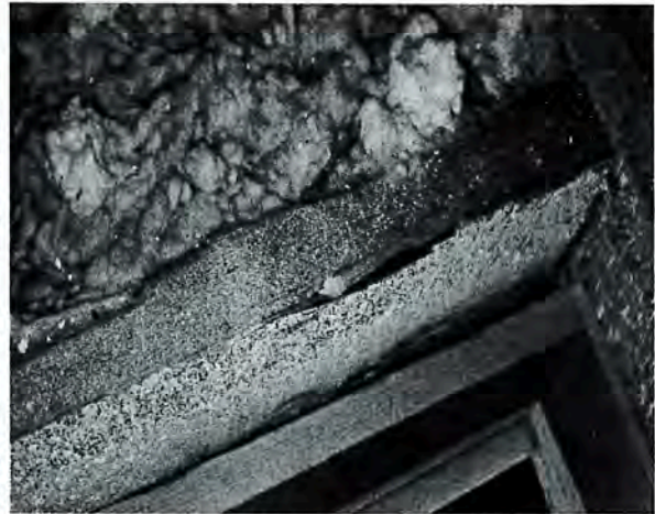
Photograph 14: Unit 206. Termites infestation
