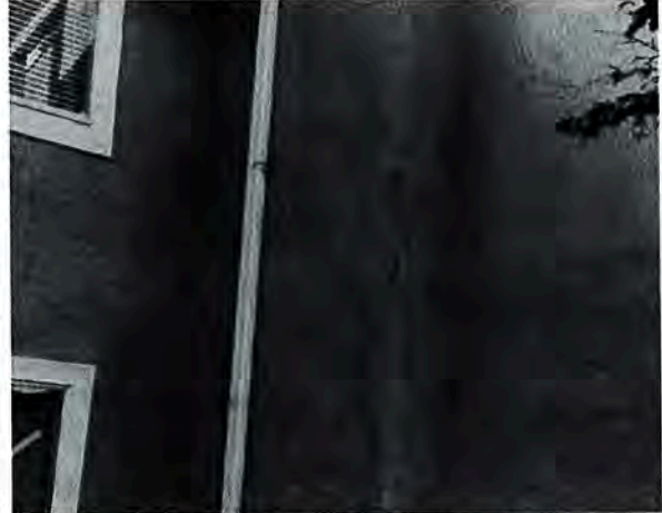
Photograph 14: Cracks on the exterior walls
