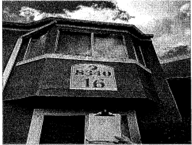
Photograph 8: Unit 107. Shoring required
