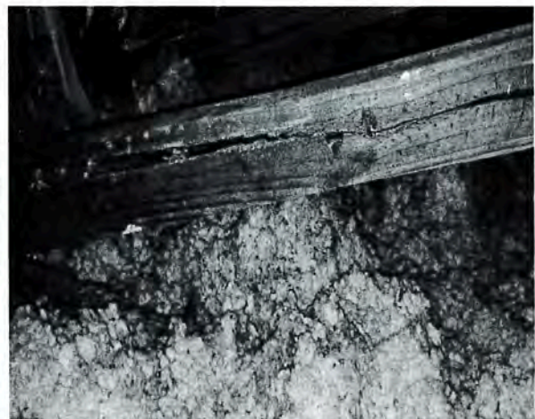
Photograph 10: Unit 202. Isolated damage to roof truss
