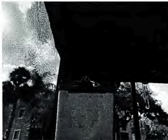
Photograph 13: Unit 106. Shoring required
