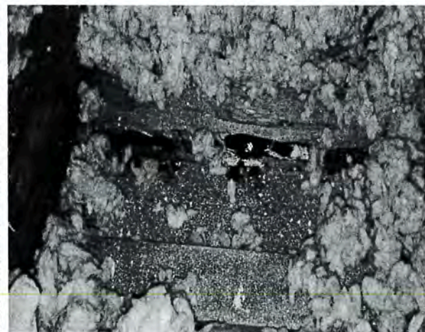
Photograph 12: Unit 208. Termites infestation
