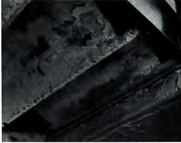
Photograph 13: Exterior staircase. Spalling and cracks
