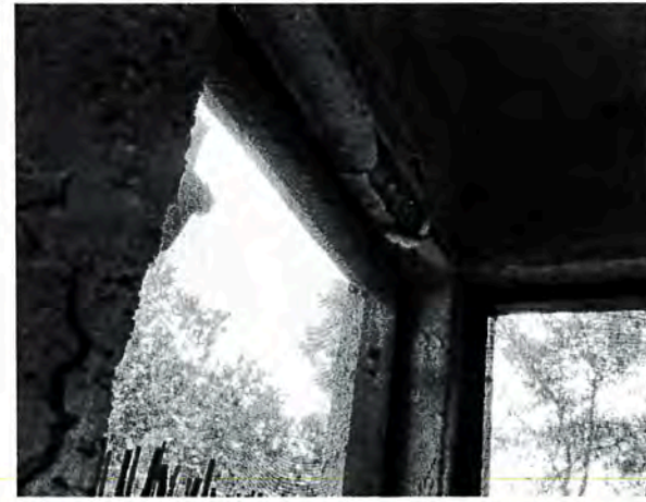
Photograph 12: Exposed wire lath on Unit 204 balcony
