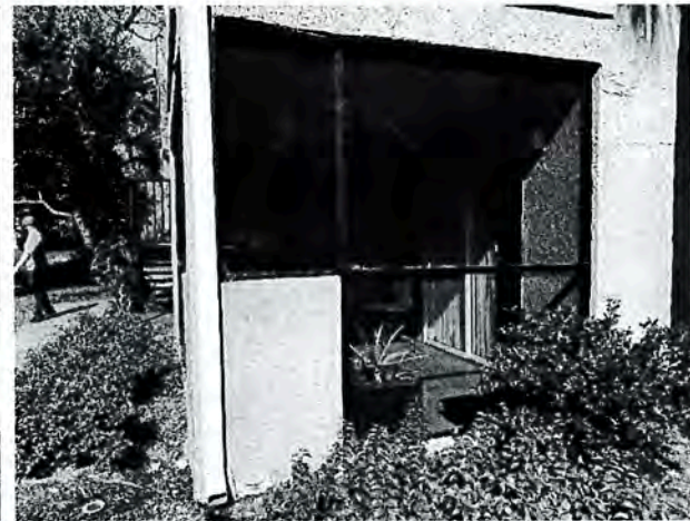
Photograph 14: Unit 106. Shoring required
