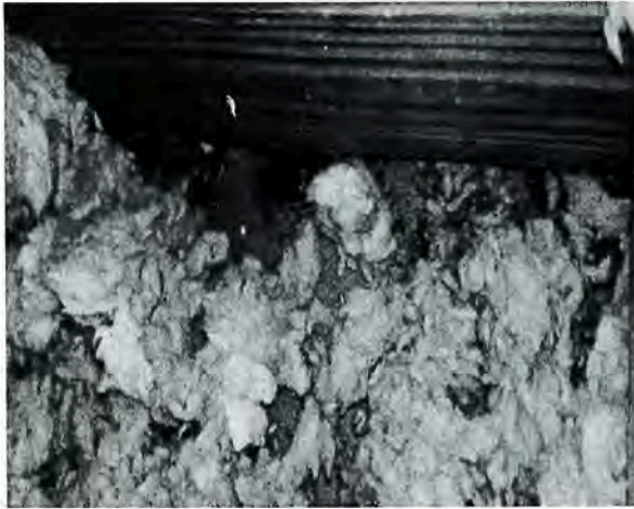
Photograph 13: Unit 205. Termites infestation
