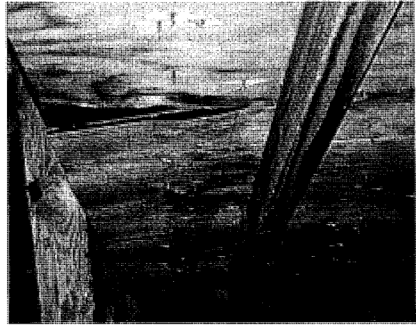
Photograph 14: Unit 203. Moisture stains and cracked sheathing in the attic.
