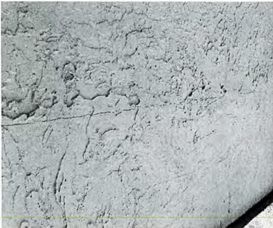
Photograph 11: Cracks on balcony ceiling Unit 104
