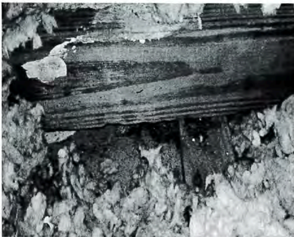
Photograph 9: Unit 201. Termites infestation
