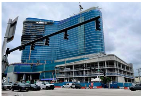
The Omni Hotel and the convention center at 1950 Eisenhower Blvd. undergoes construction in January. Broward County approved hiring an asset manager to keep tabs on the project. MIKE STOCKER/SOUTH FLORIDA SUN SENTINEL
